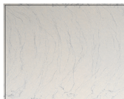
COVERAGE TOO LIGHT
